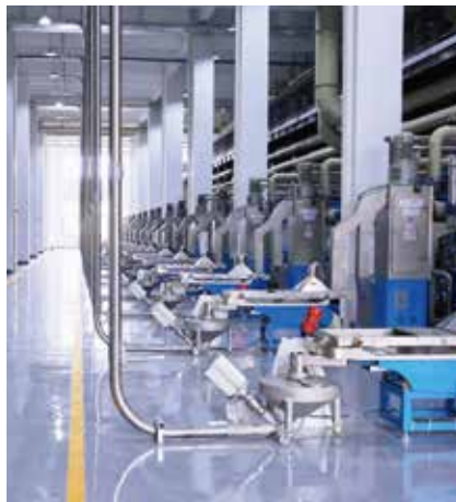
原料改性车间 Compostable Material Modifying Workshop
