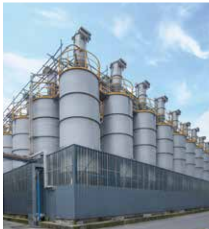
数字化配料系统 Digital Compounding System
